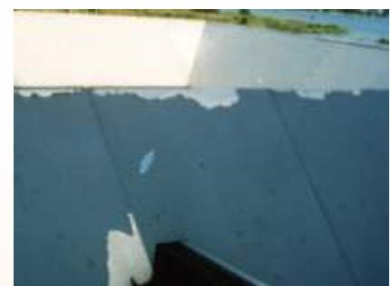
Img. 5.3.3. Blistering caused by cross-linkage
