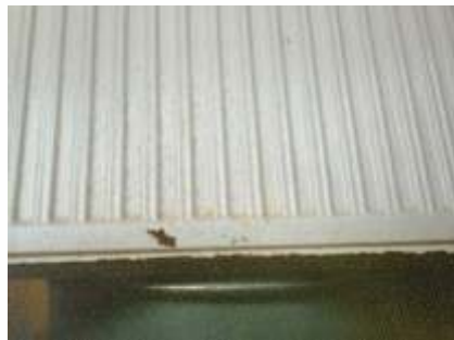
Img. 4.1.2. Infiltration caused by chemical exposure
