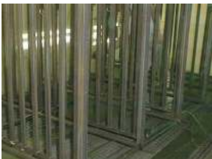
Img. 2.4.1. Corrosion as bubble causale
