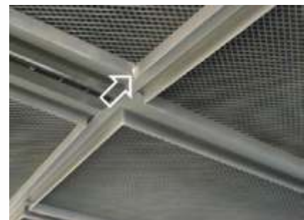
Img. 6.4.3. Sweat-cinder not removed
