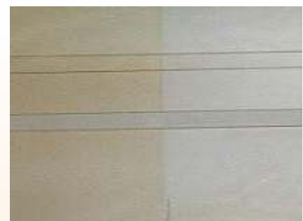
Img. 3.2.3. Yellowing in the interior caused by UV-light
