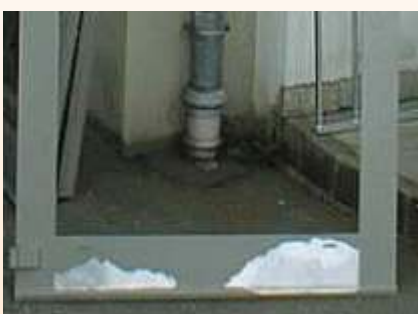
Img. 5.3.4. Blistering caused by an inappropriate pretreatment
