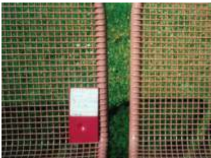
Img. 4.1.1. Chalking caused by faulty powder coating selection
